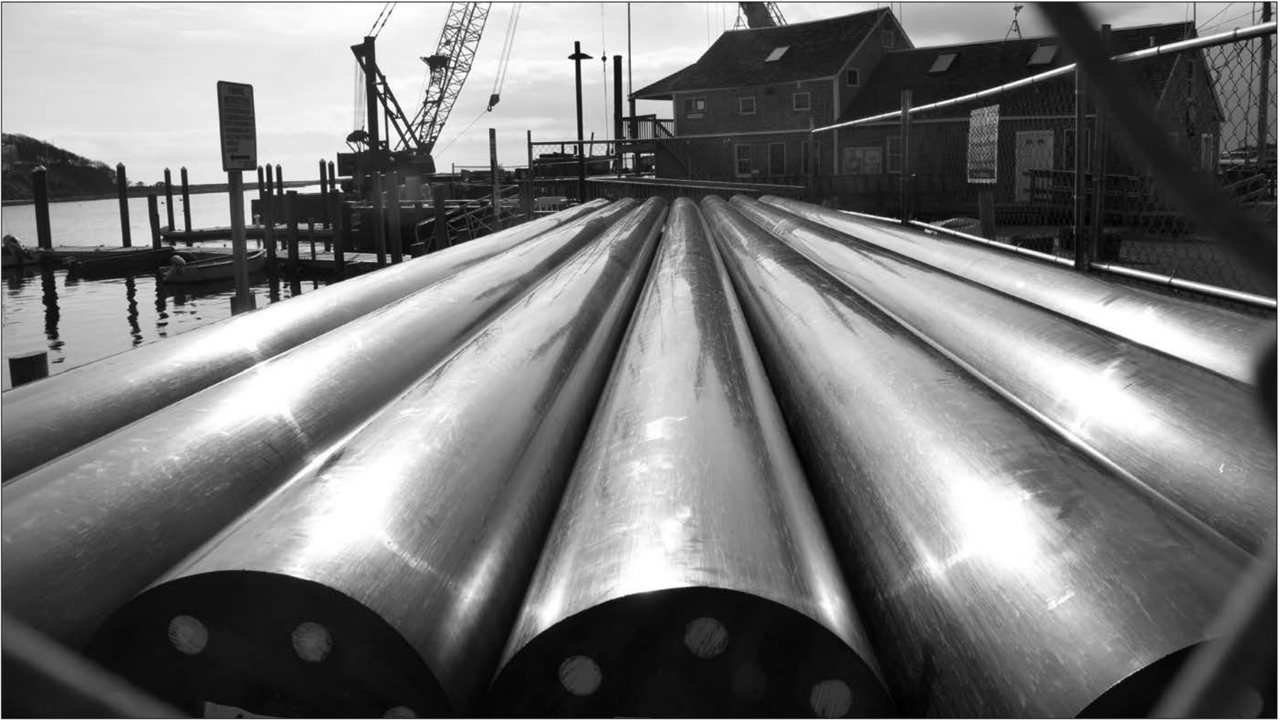
Pilings await installation as part of the renovated trap dock on Stage Harbor. TIM WOOD PHOTO
